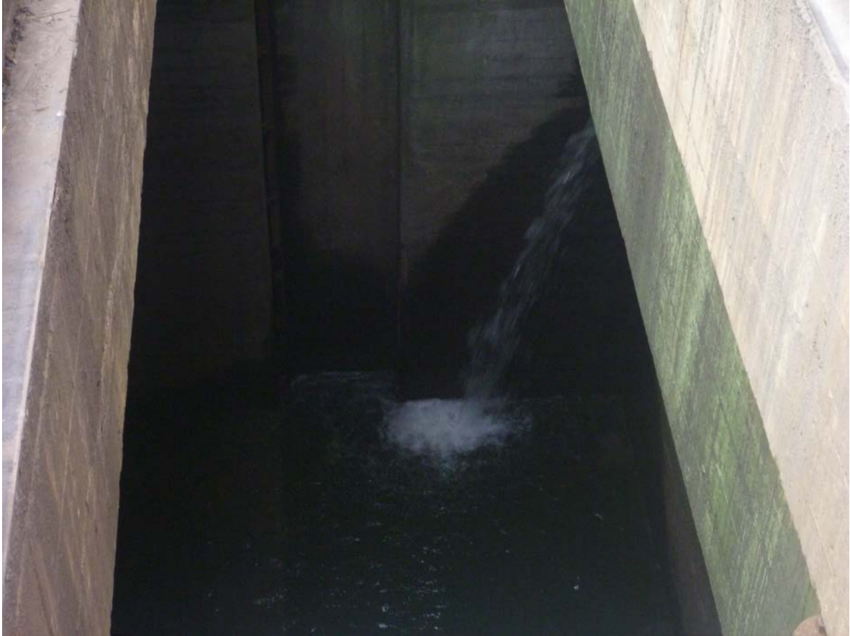
Figure 1. Unit 8 tail log slot cooling water discharge from above, looking north. This discharge has only been running since 20 June.
